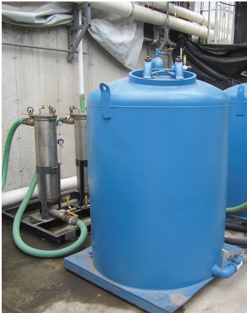
Figure 4. A GAC filter being tested in a commercial location. A pre-filter takes out suspended particles. GAC packed into rapid-sand filters then removes agrichemical residues.
